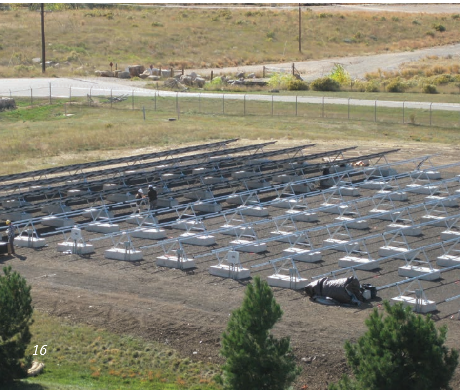
Solar farm at City's Water Treatment Plant
